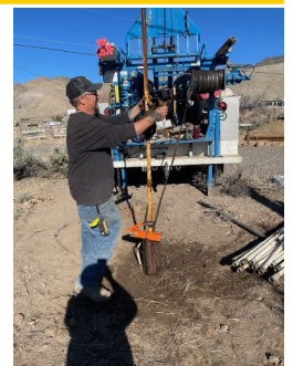
Pump Coming Up
