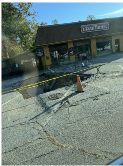
Parking Lot Sinkhole
