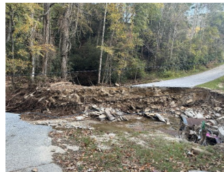
Washed Out Road
